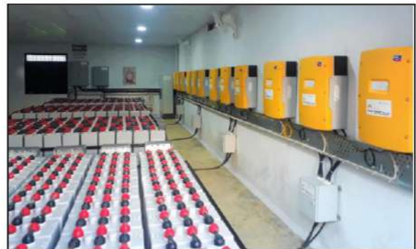
Figure 8: Battery bank and inverters inside powerhouse
